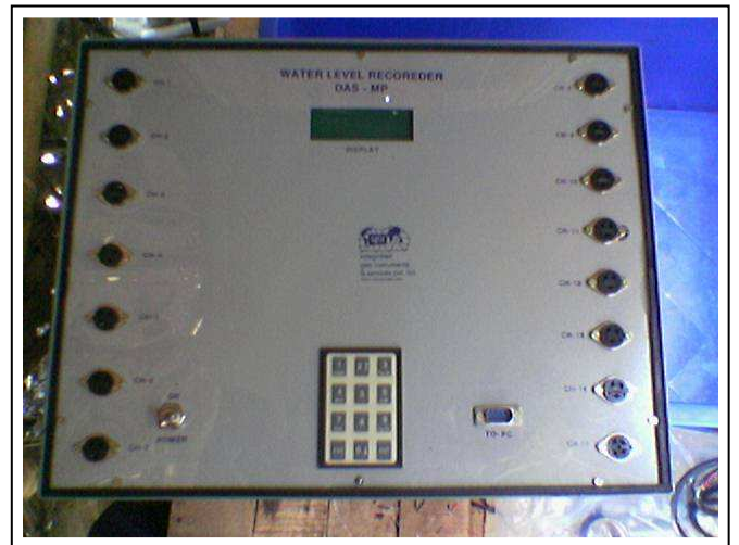
15-channel Water Level Recorder with built-in micro-processor and embedded software to record the water levels at 10 minute interval, store the data in memory and also transmit the data through telemetric system to be accessed anywhere in the world.
